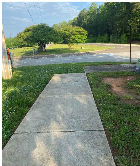
End of sidewalk at the eastern driveway
